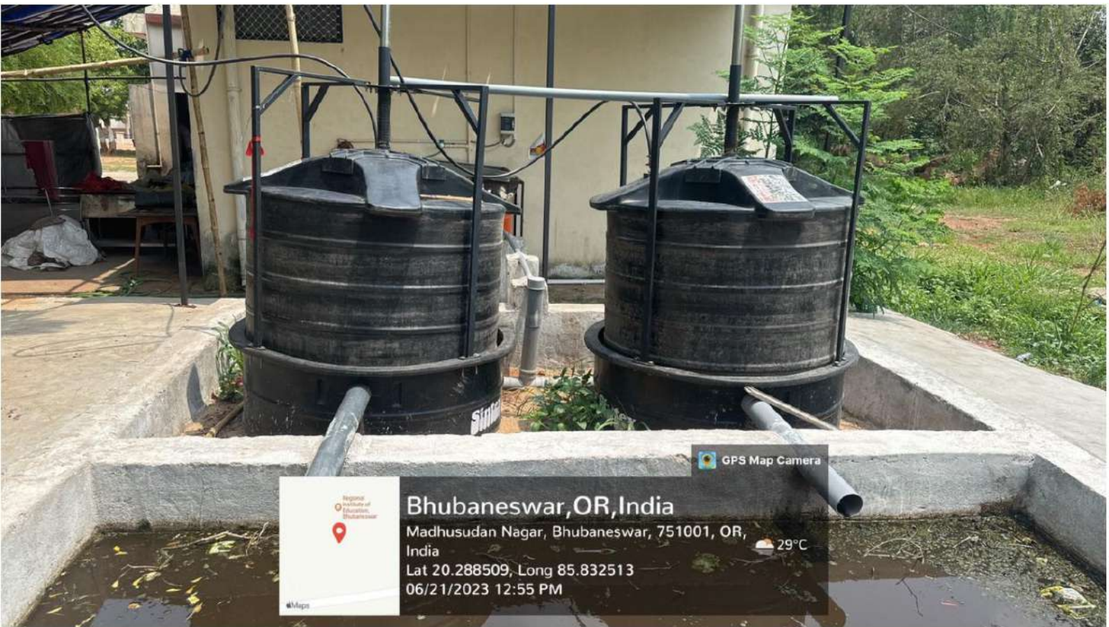
BIO GAS PLANT REGIONAL INSTITUTE OF EDUCATION ,BHUBANESWAR
