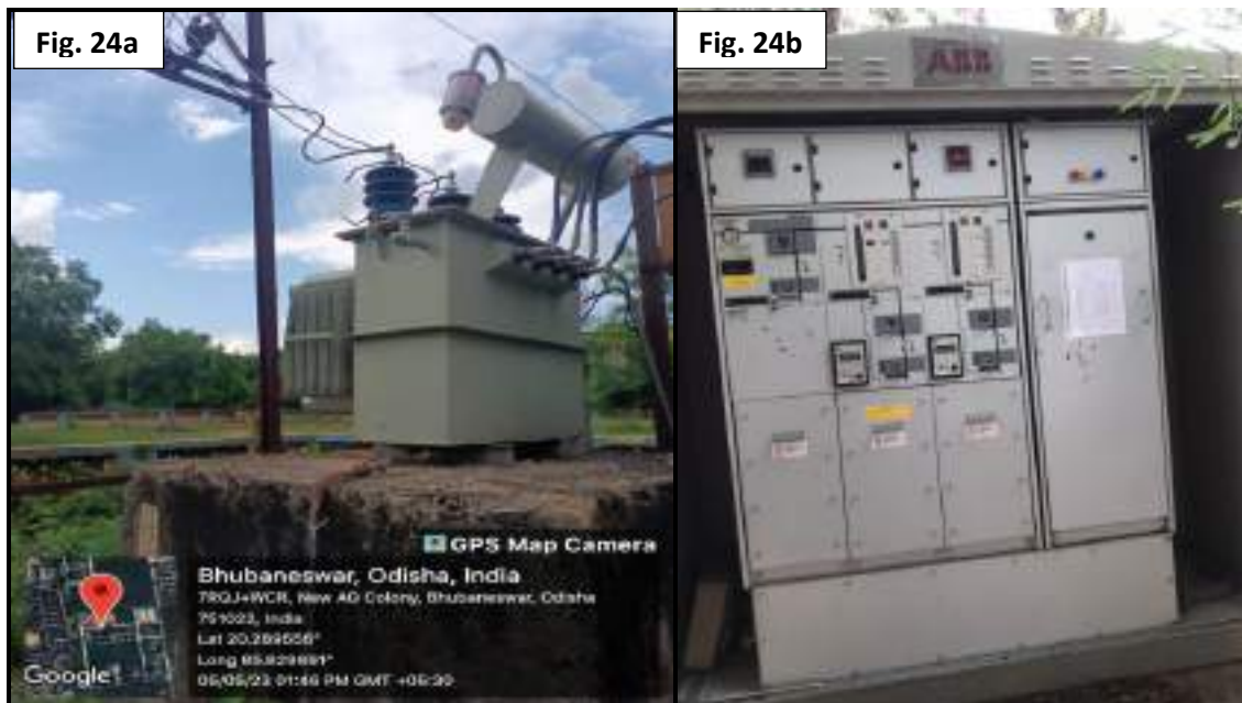
Fig. 24(a-b) – Transformer Installed in the Residential Area and Institute
