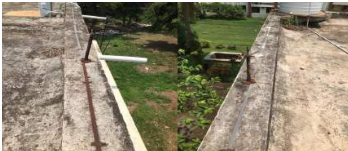
Fig. 50 – Lightning Arrestors in the Terrace of Institute’s Main Building and D.M.School Building
