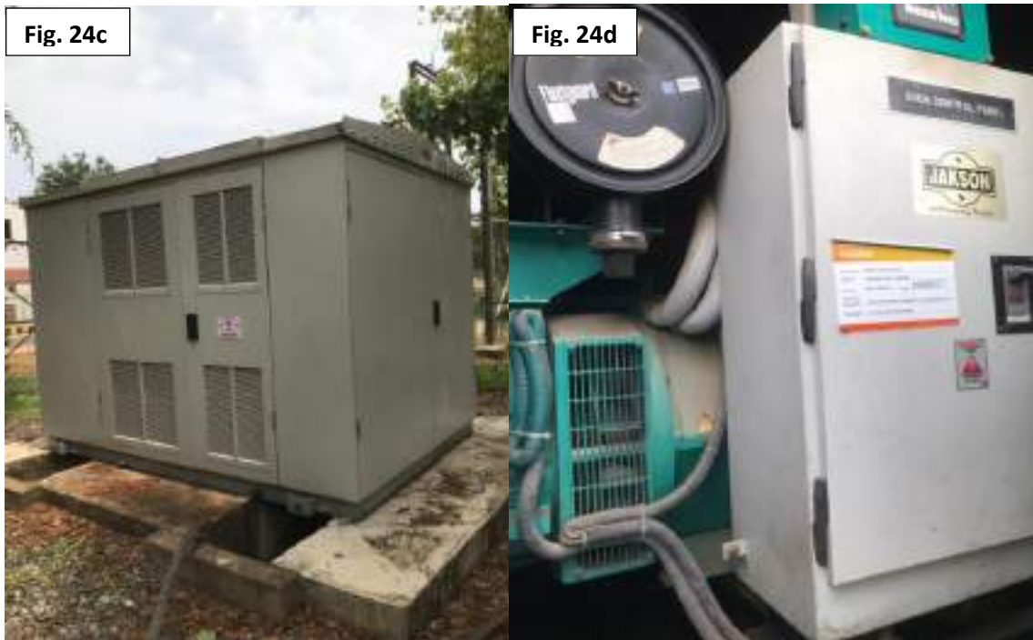
Fig. 24(a-b) – Transformer and DG Installed in the Institute.
